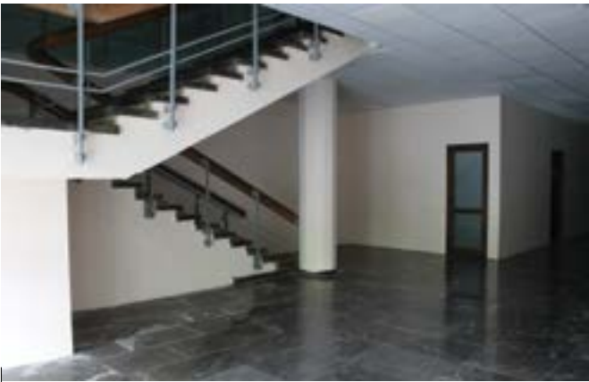
Tuff tiles cladding of the column covered with paint layer. 2018
