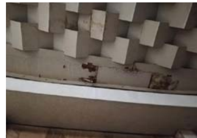
Fig. 21 The suspended ceiling in the Main Hall, damaged by roof leaks
